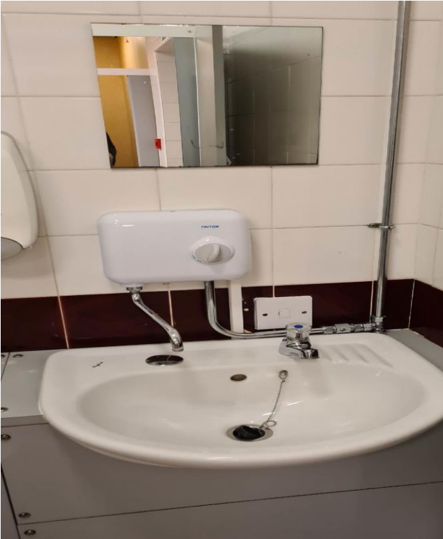
POU Water Heater
